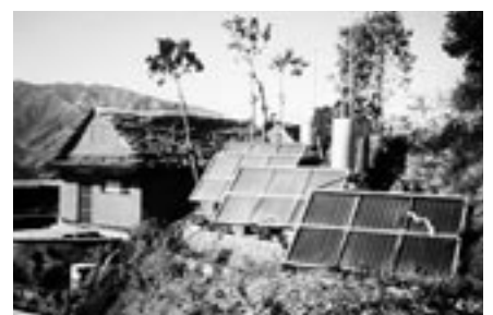
Fig. 13b: Solar water and space heating in Kathmandu, Nepal. Photograph by Dr. Donald Aitken
